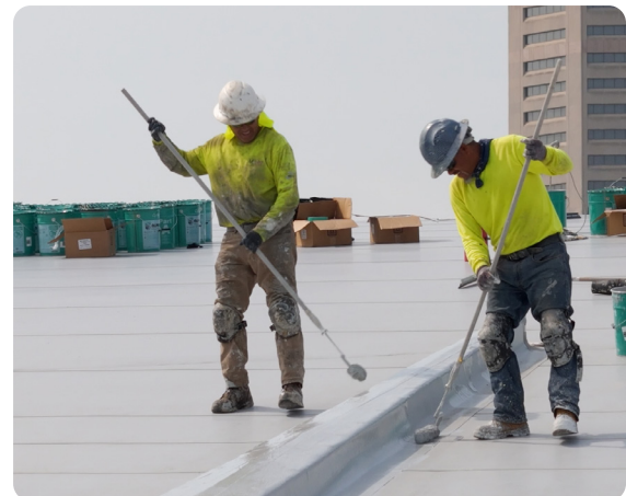
AlphaGuard PUMA Top Coat is applied to provide the building a long lasting durable roof finish
