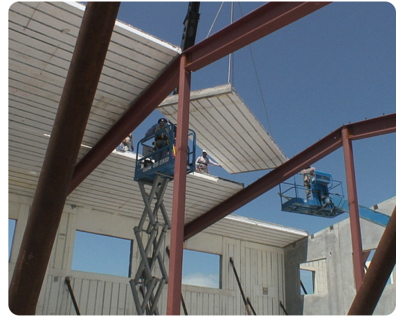
Nadura Deck Forms are lifted by crane and installed spanning the buildings steel joists
