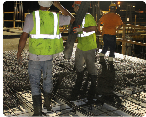
Concrete is poured and prepared to meet the ICRI profile rating specified for the project
